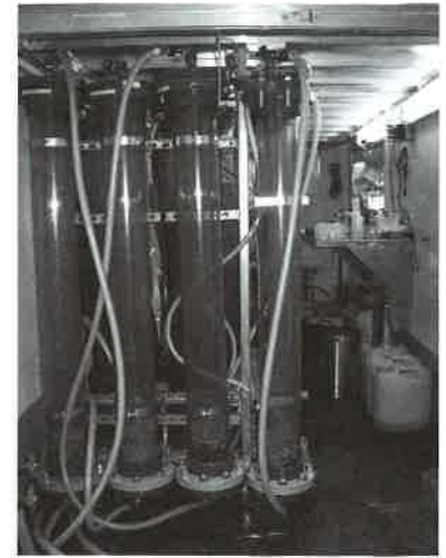
Filtration columns at the Kennedy Pilot Treatment Plant in North Acton.
